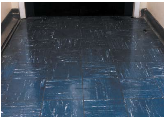
Figure 48e Asbestos-containing vinyl floor tiles
