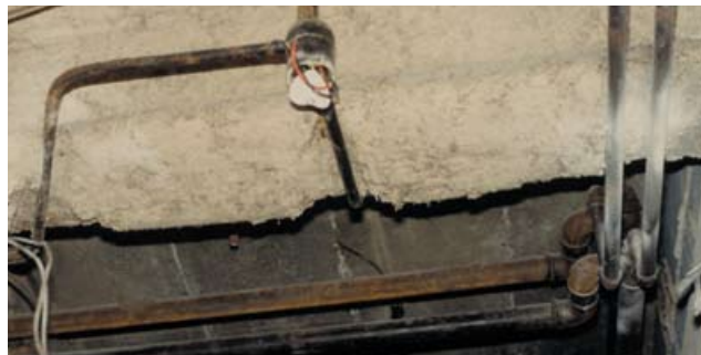
Figure 48b Poorly tamped sprayed chrysotile fireproofing on a structural steel beam holding up a concrete floor, showing some overspray onto the concrete and damage by electrical work
